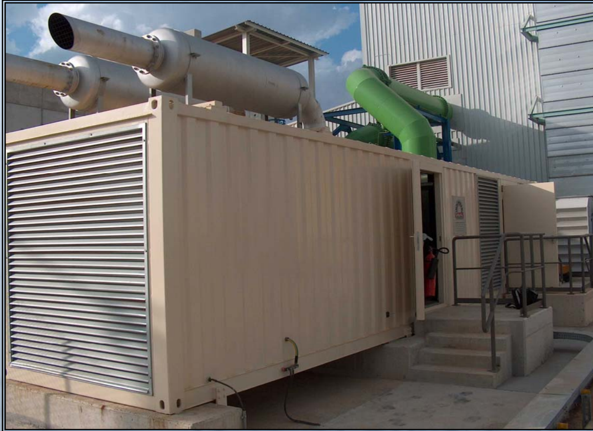
Containerized Modules with MTU 16V 4000 Engine for Emergency Power Supply
