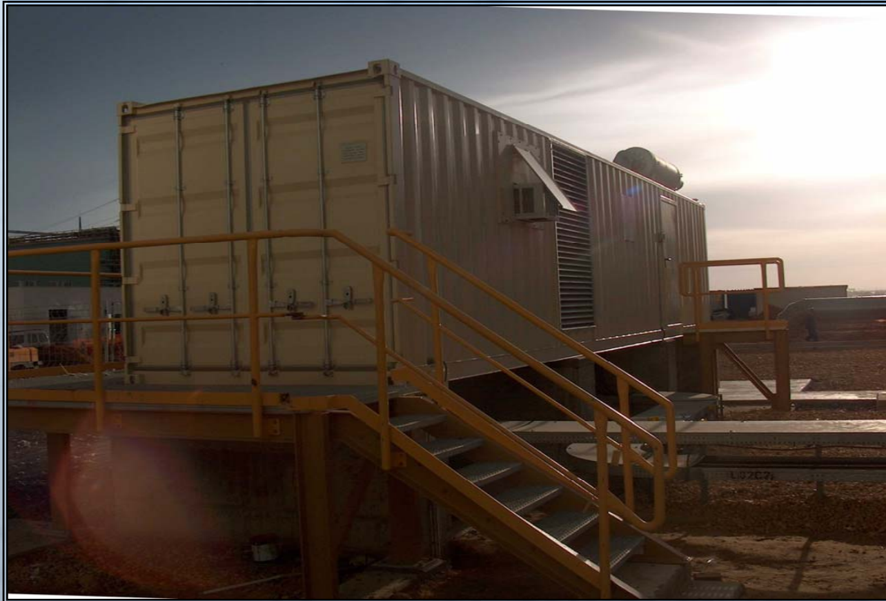
Containerized Modules with MTU 16V 4000 Engine for Emergency Power Supply
