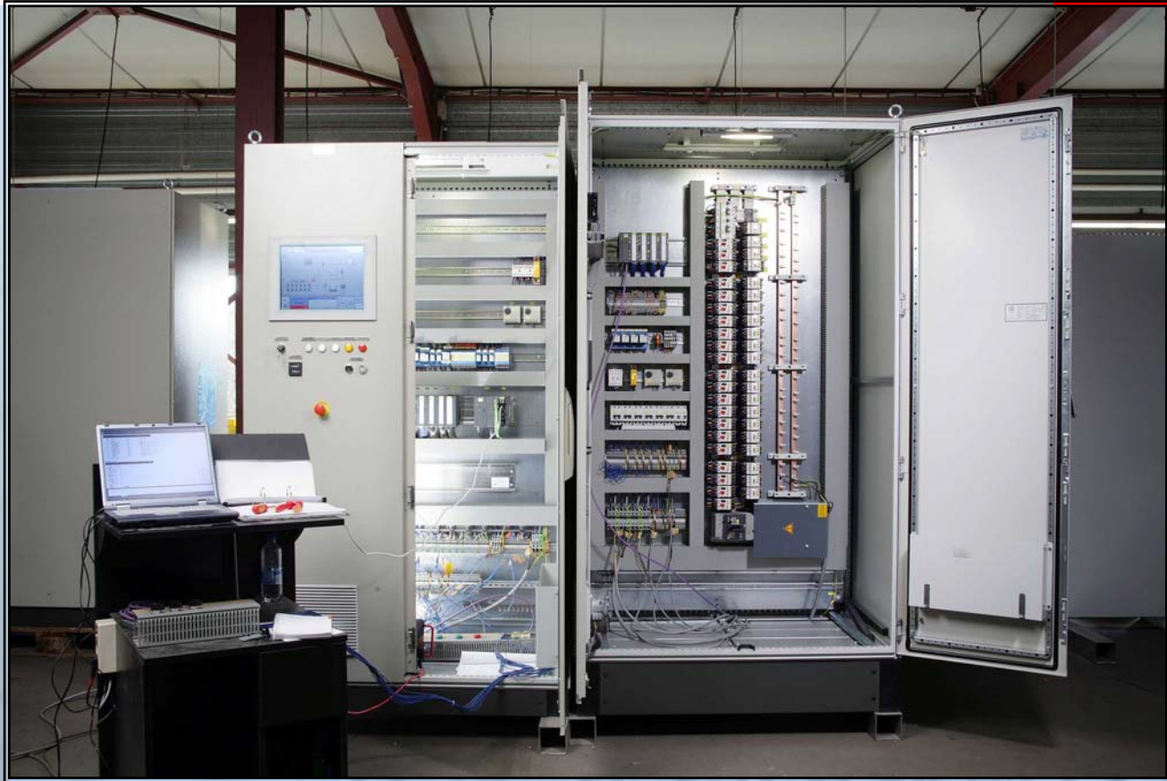
Switchboard for Pipeline-Pump (Sudan, Africa)
