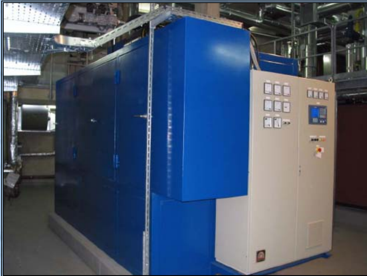
CHP for Swimming Pool in Germany (386 kW, MAN)
