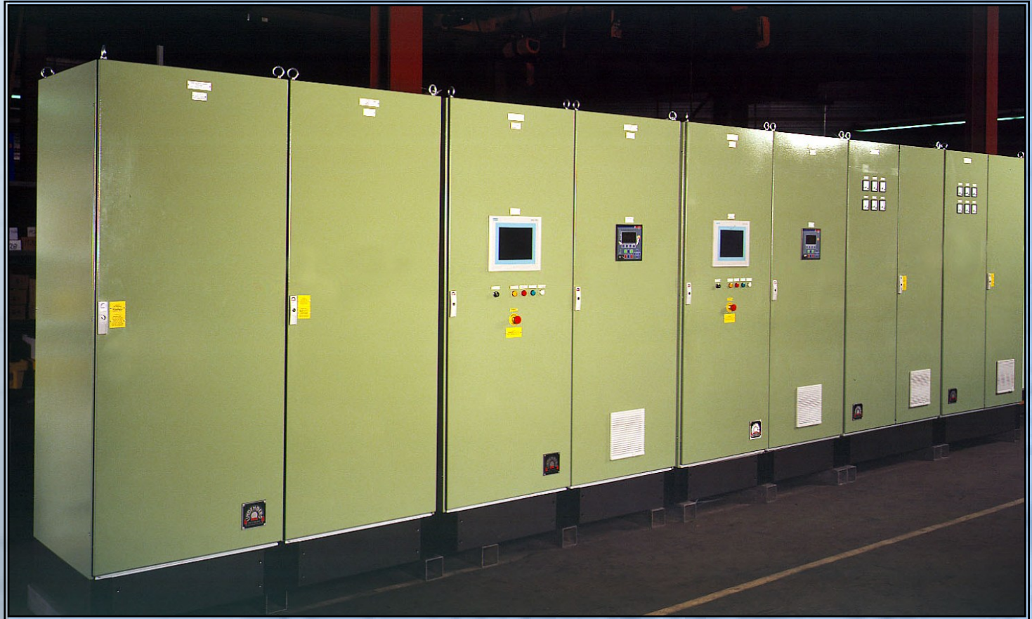
Switchboards for Krupp-Uhde
