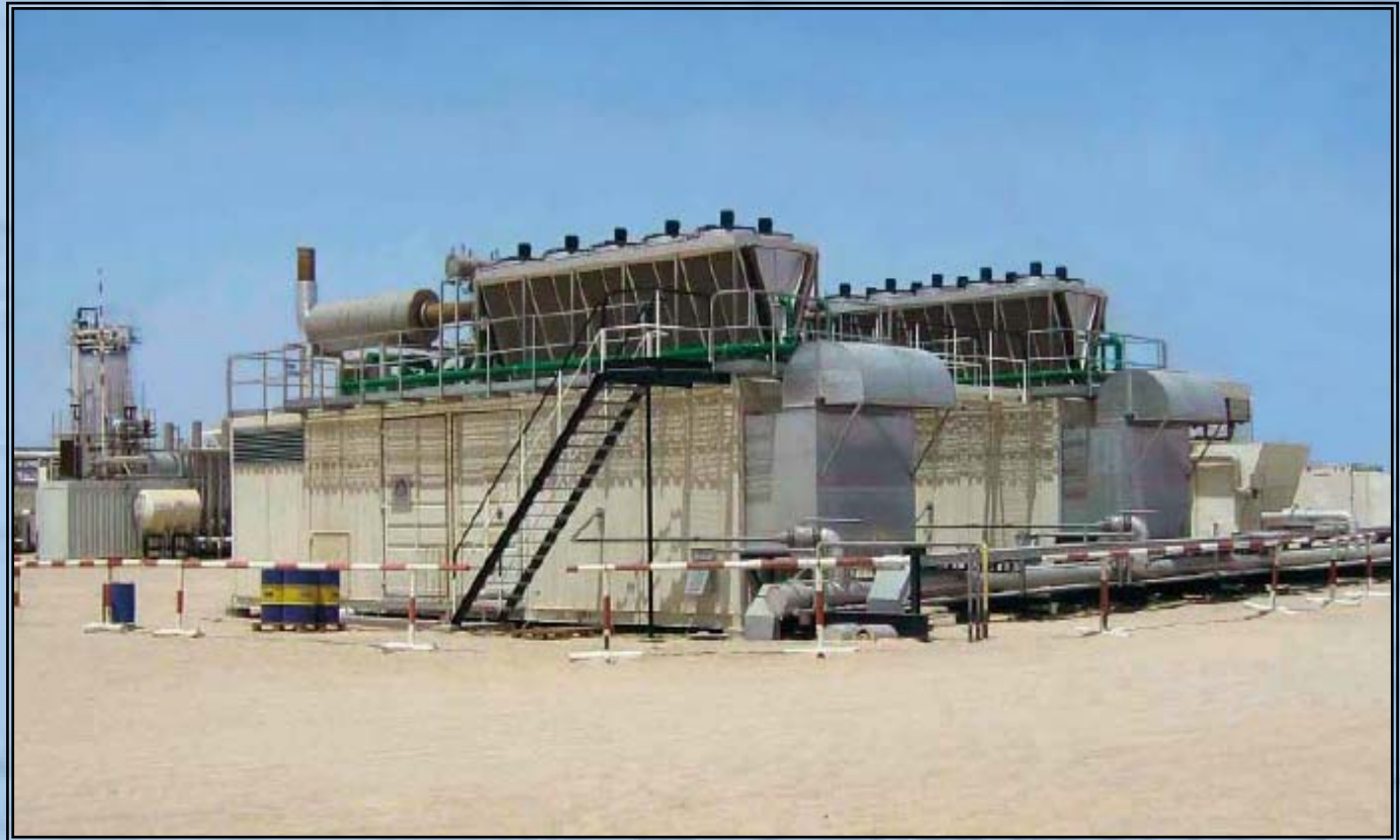
Containerized Gas Gensets 2 x 1,2 MW (Waukesha) for Wintershall (Germany); Power Supply for Oil Field in Libya
