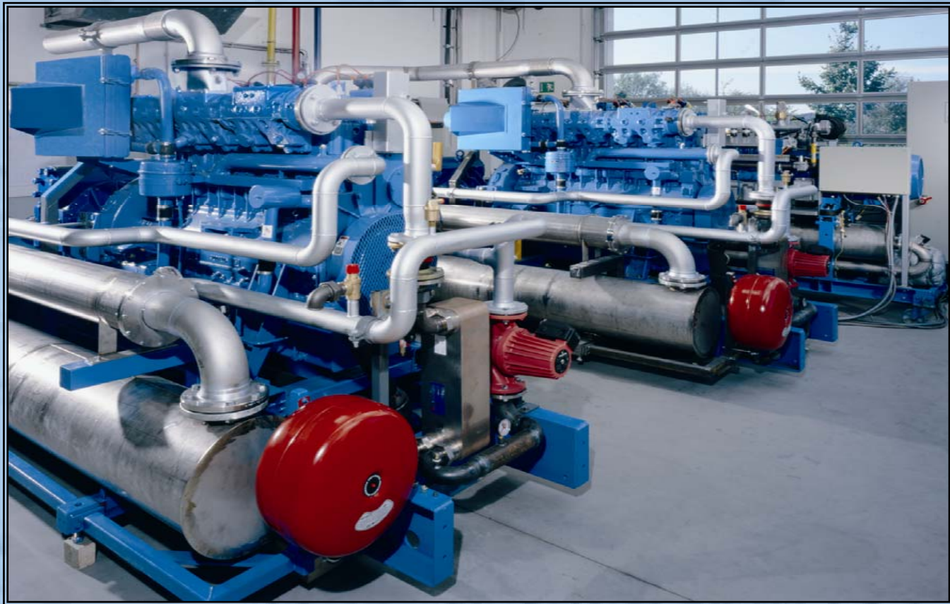
Compressor Drive for Heat Pump in Germany (Waukesha)
